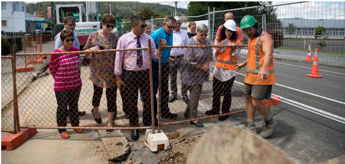
Briefing new councillors and the Mayor of Porirua City Council, Mike Tana, at an Upper Hutt wastewater pipe renewal site
