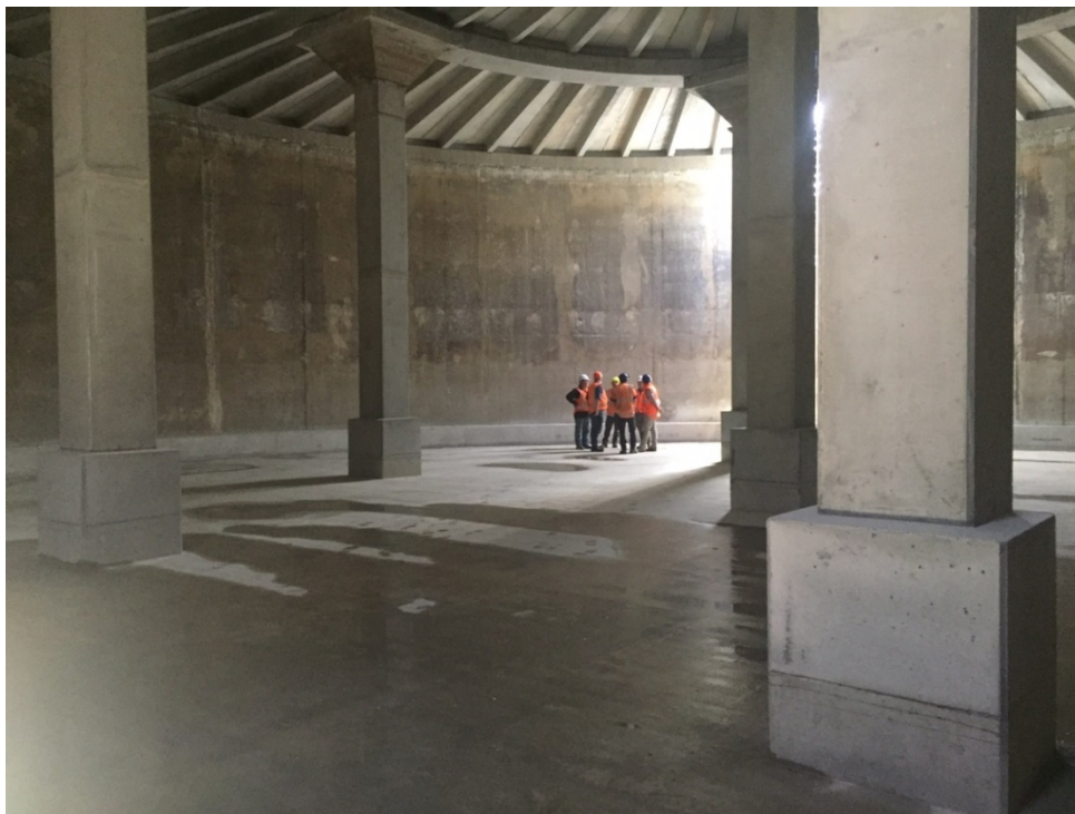
Inside the Konini Reservoir in Wainuiomata where we carried out earthquake strengthening.
