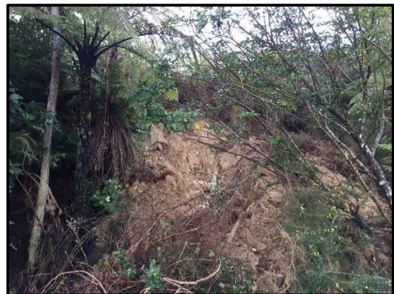
Photo 6: Recent instability on a previously cut slope at the toe of the hills.
