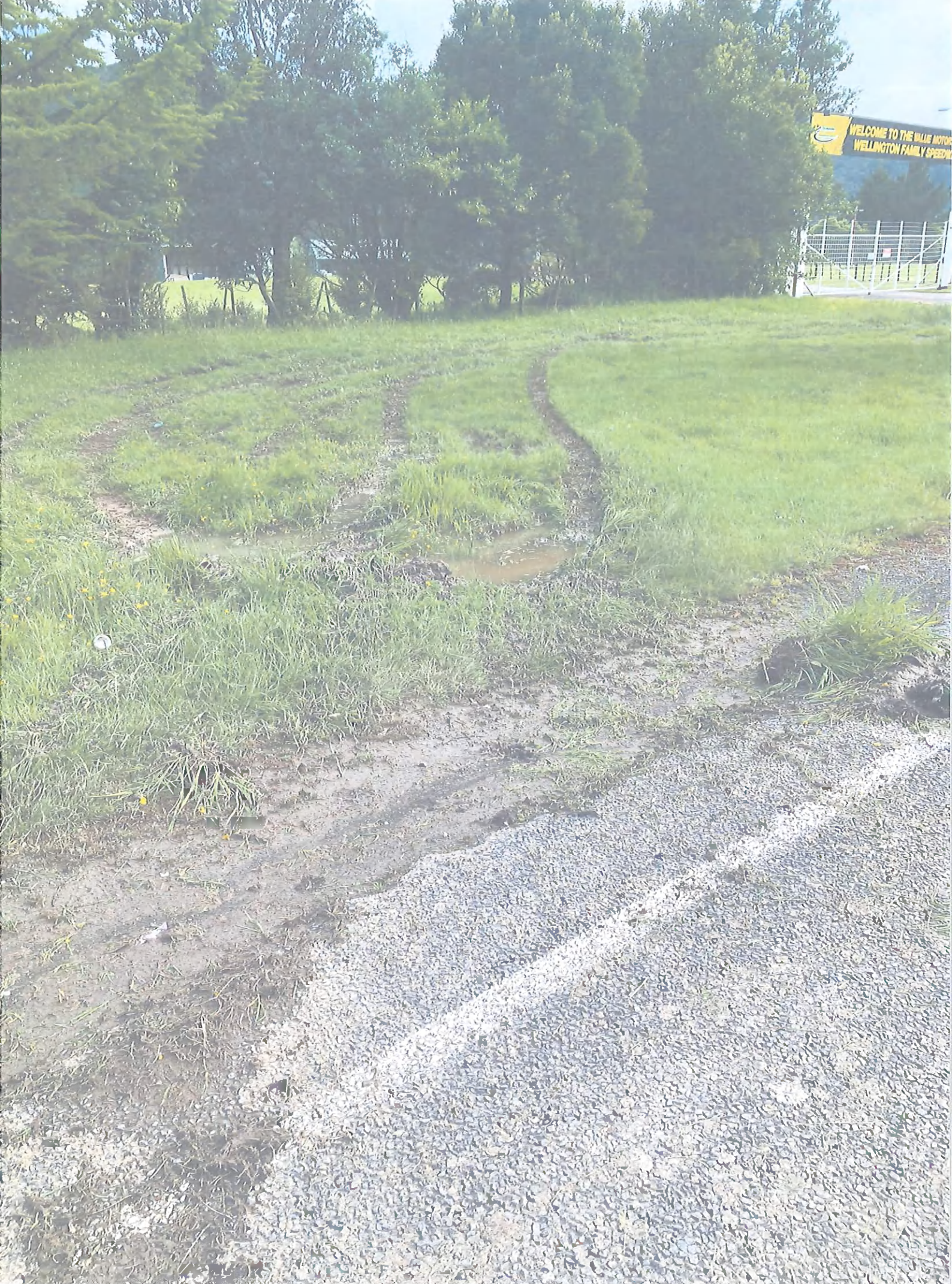
Damage done by racers on Burn. Twin Lakes Rd
