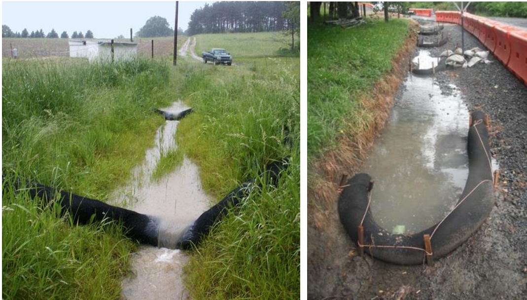
Figure 13: Example Photo of Filter Socks
