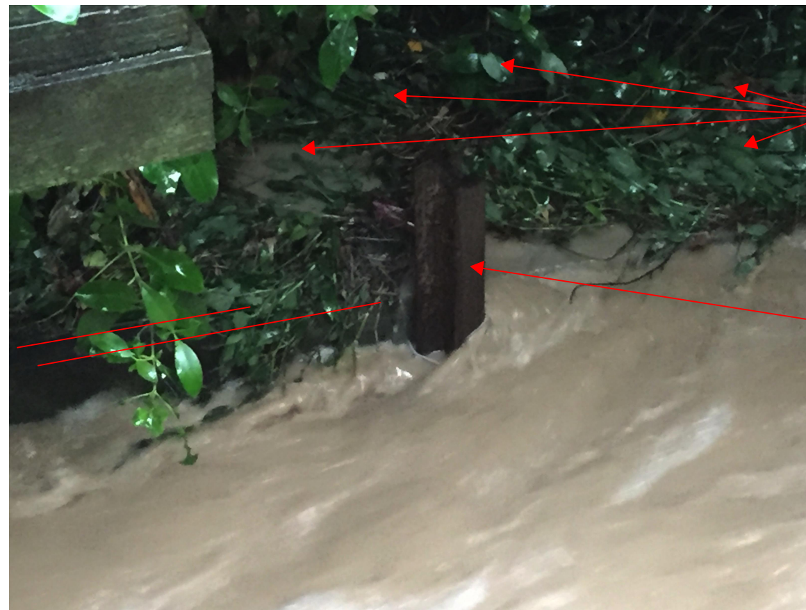
4 - Right Bank at Retaining Wall post (about 1.8m upstream of weir) 7:18am
