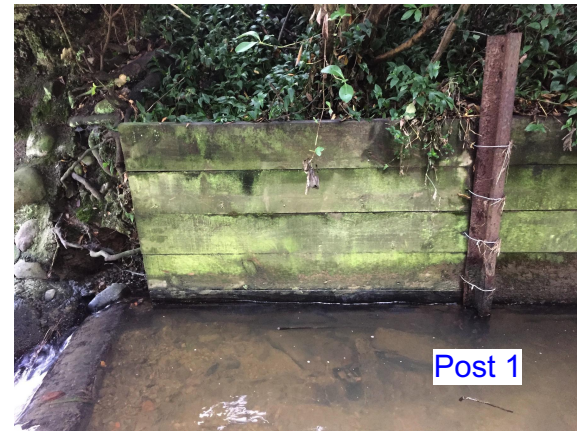
6 - Railway iron at retaining wall
