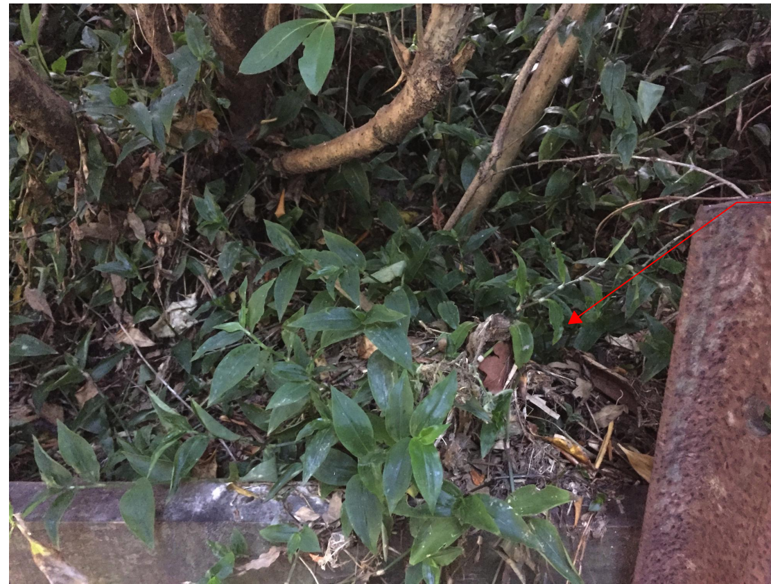
2 - Debris still evident 16/3/20 above retaining wall and at base of tree.
