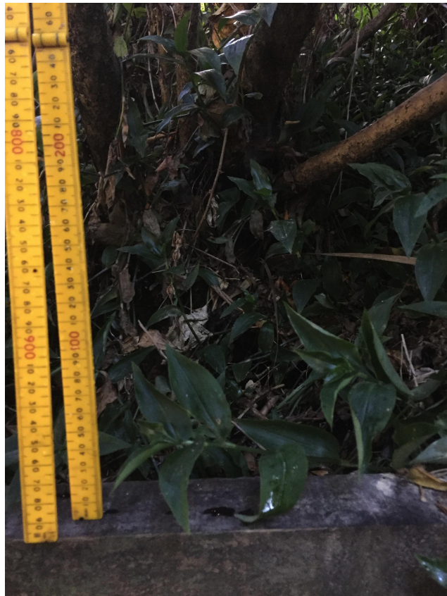
1 - Debris 100mm to 150mm above top of retaining wall.
