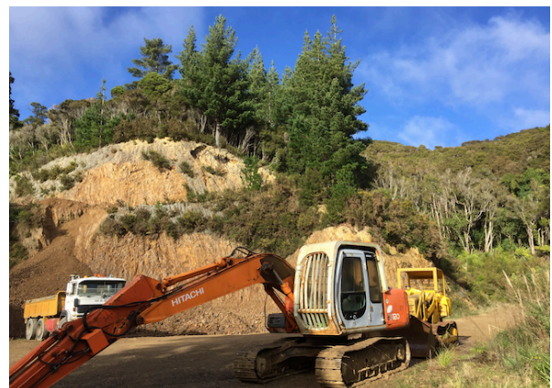
Figure A6 - Quarry on sub-catchment B
