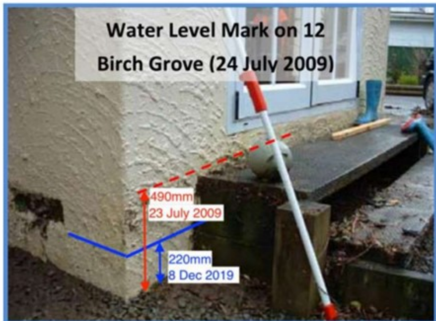
12 Birch Grove – 23 July 2009 flood was bigger than 8 December 2019 flood.
