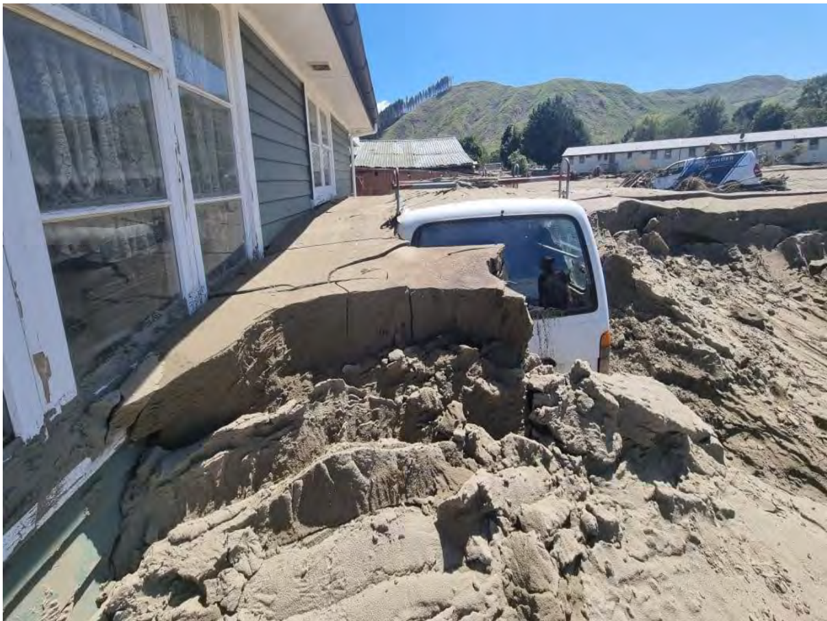
Flood damage in the Esk Valley in Hawke's Bay after Cyclone Gabrielle. Photo: RNZ / Tess Brunton
