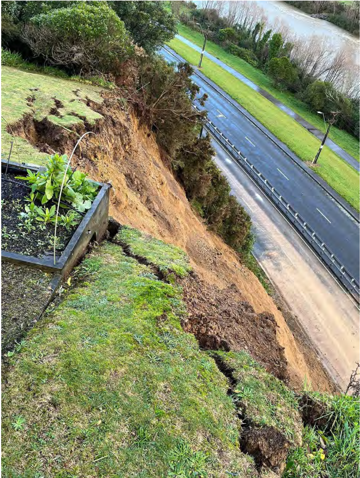
Two planter boxes have been written off due to their proximity to the edge of the slip. Photo / Supplied In Wellington, the main route into the suburb of Wadestown is also cut off, and will likely remain so until early next week.
