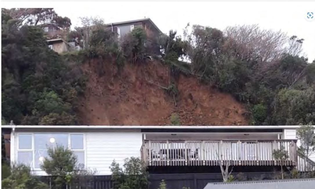
The slip on Wednesday morning left a house near the edge. Photo credit: RNZ/Kevin McCarthy
