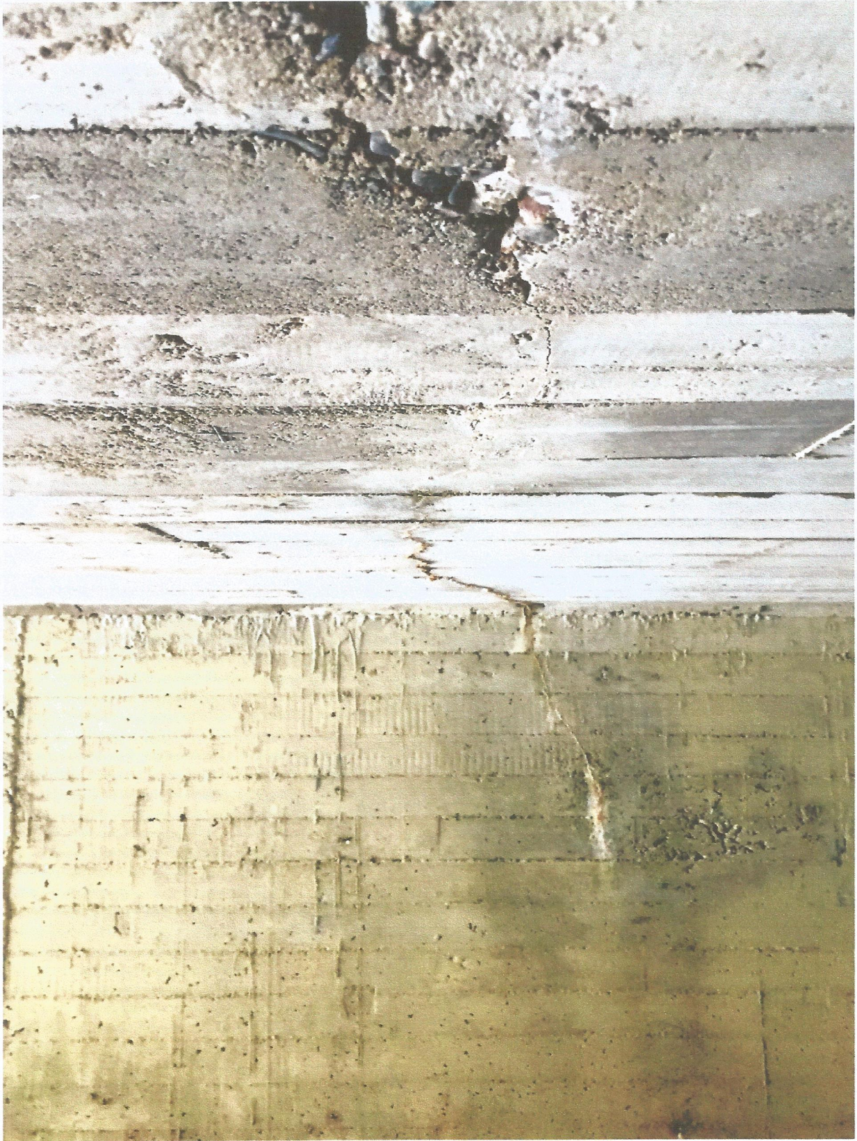
Soffit crack showing honeycomb and efflorescence
