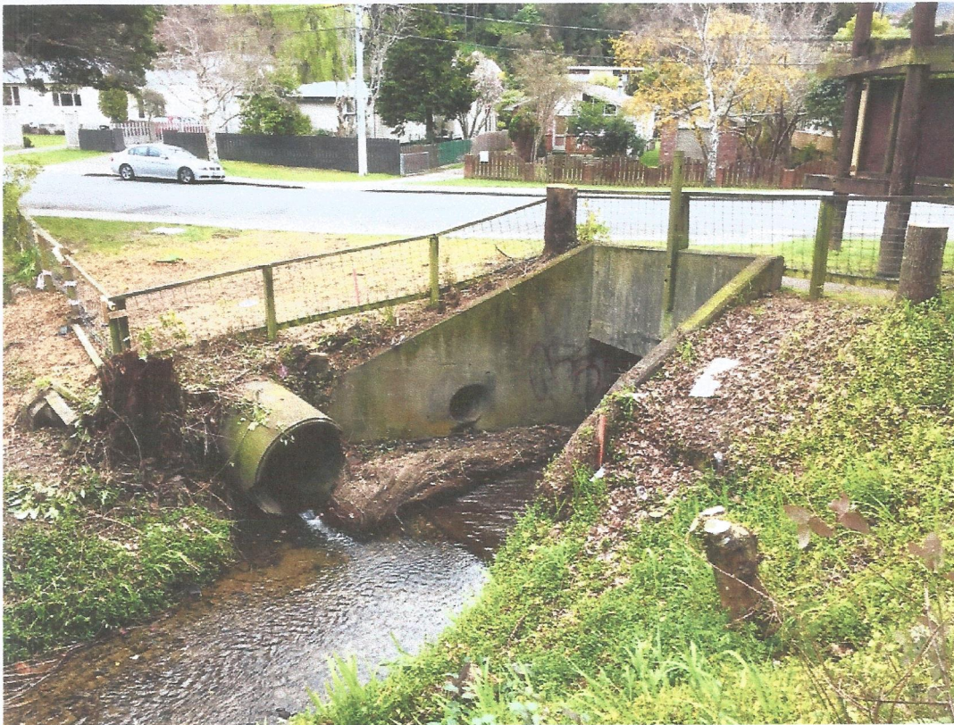
Inlet showing debris build up and scour underneath large pipe
