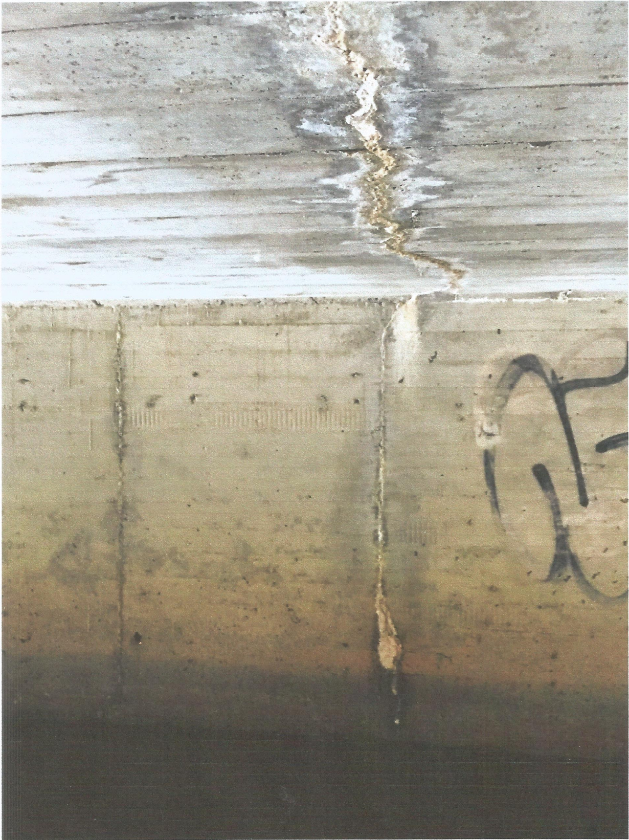
Crack 2 showing efflorescence and graffiti
