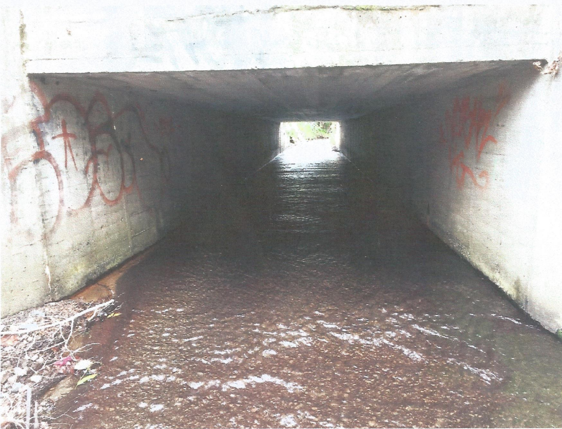
Inlet showing graffiti
