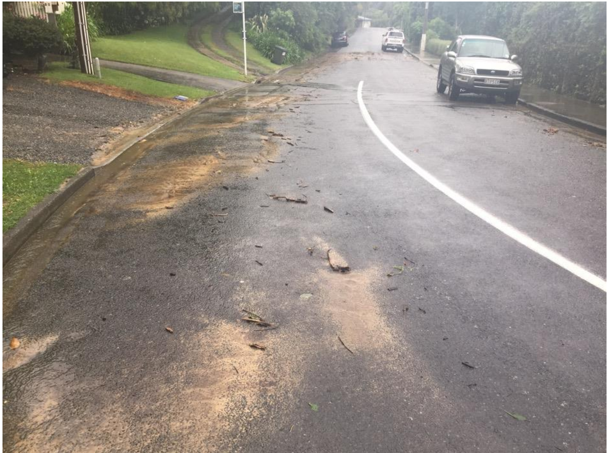
Jocelyn Crescent – due to overtopping of culvert at 122 Pinehaven Road
