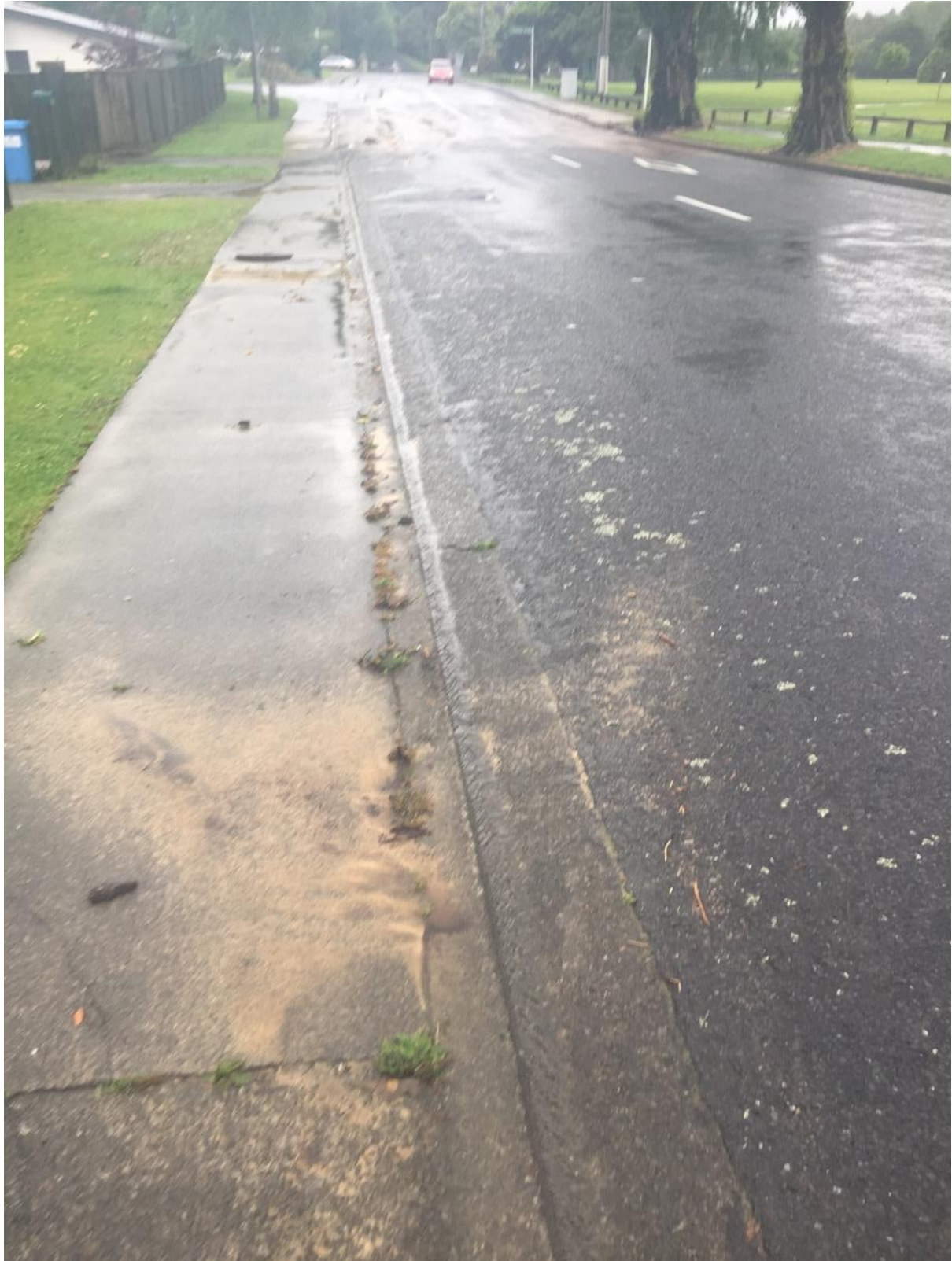
Pinehaven Road – (opposite Pinehaven School), 09:26 am – due to overtopping of driveway culvert at 122 Pinehaven Road.
