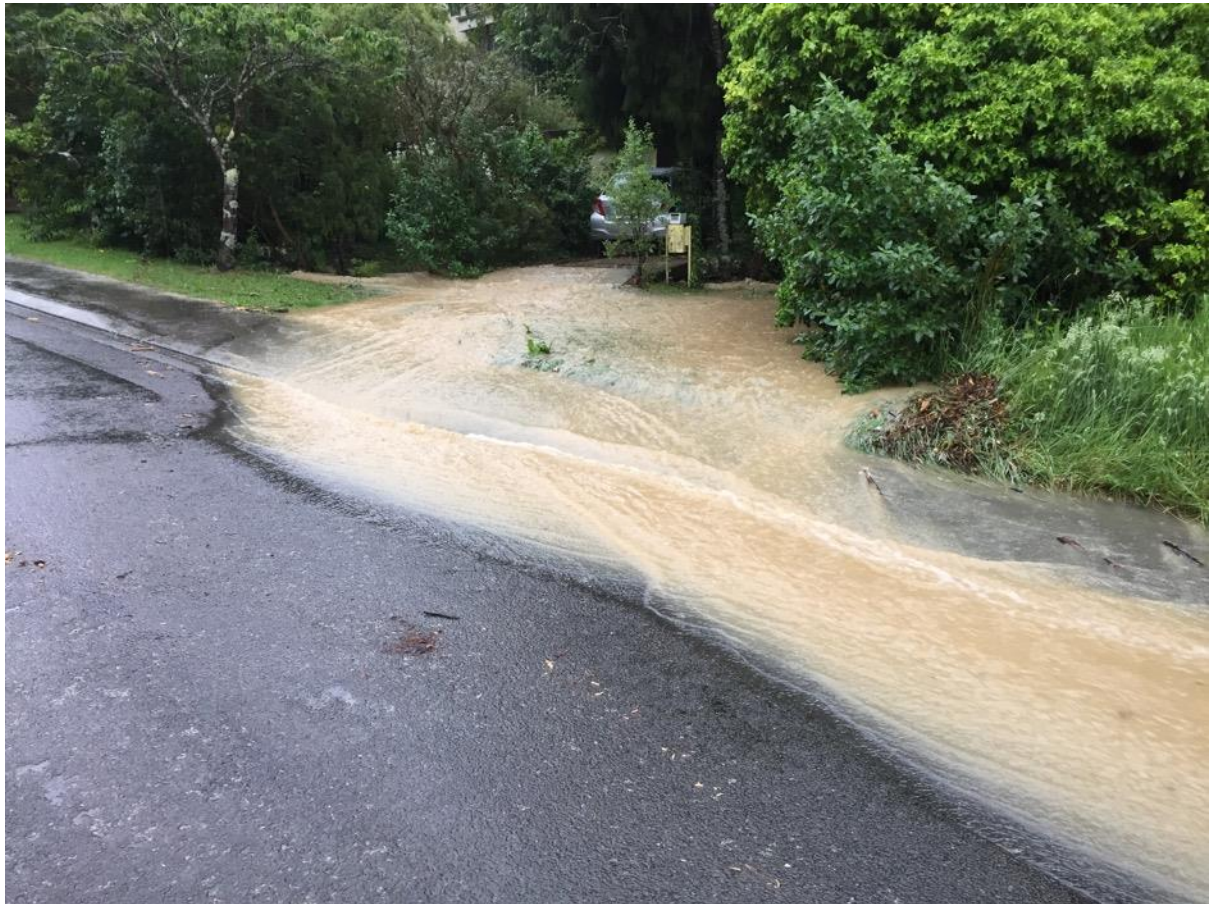
122 Pinehaven Road, overtopping of driveway culvert, 05:05 pm (mid-afternoon rain)
