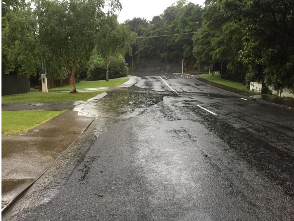
06:45 am – ponding due to blocked sump
